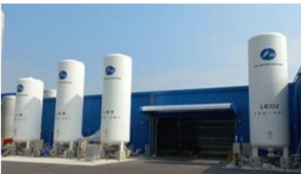
CE (Low Temperature Liquefied Gas Storage Tank)
