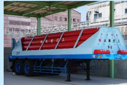
Cylinder bundle device of hydrogen gas
