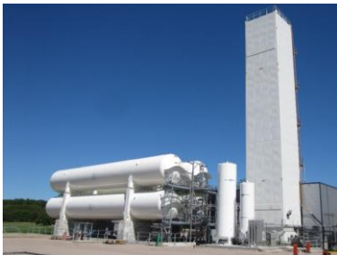
Cryogenic air separator
