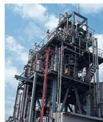
Liquid-phase air oxidation system
