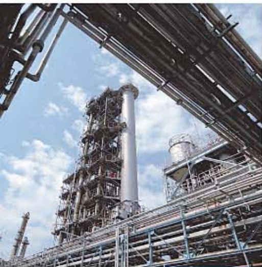
Tar distillation plant at the Kashima Plant
