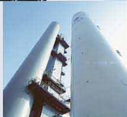
Wakayama Plant Air Separation Plant No. 12
