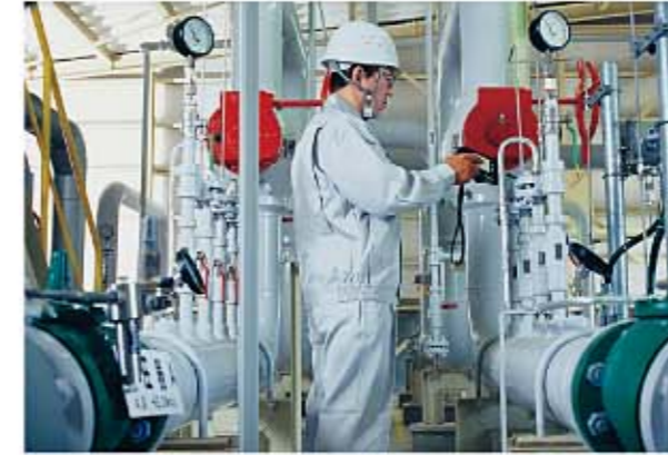
Natural gas supply system
