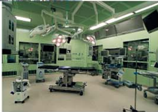
Operating room equipment
