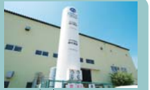
Artificial air generating systems
