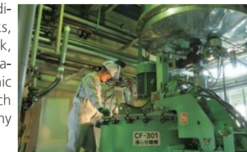
Fine chemical manufacturing equipment (centrifuge)
