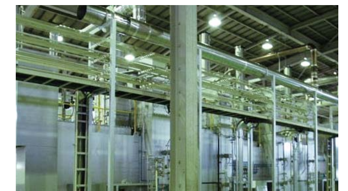
New continuous NV treatment furnace
