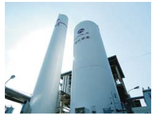
"V1" high-purity nitrogen generator
