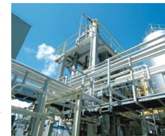
"VH" (Hydrogen Production Using Thermo-Neutral Reforming) system
