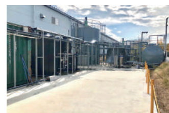
Methane fermentation demonstration plant
