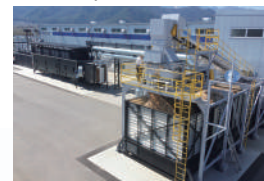
Compact woody biomass power generation plant (Azumino, Nagano Prefecture)
