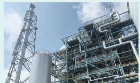
The Ako No. 2 Woody Biomass Power Station, which began operations in January 2021
