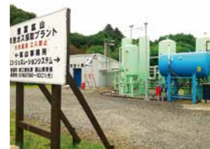
Natural gas extraction plant in Toyotomi
