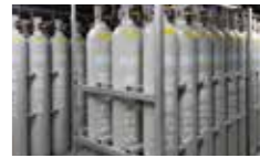
Gas fire extinguishing equipment
