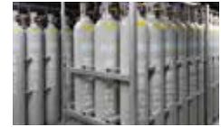
Gas fire extinguishing equipment
