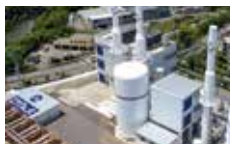
On-site gas supply
