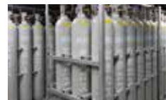
Gas fire extinguishing equipment
