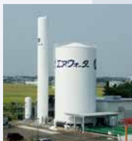
The first VSU, Niigata Ekisan
