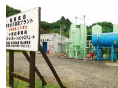
Natural gas extraction plant in Toyotomi
