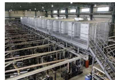
Azumino Biomass Energy Center Gasification Power Generation System
