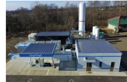
Hydrogen Farm in Shikaoi Town, Hokkaido
