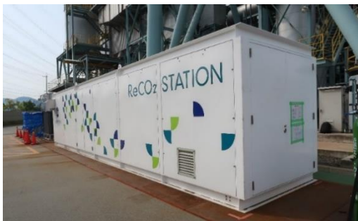
Exterior of the system installed in a power plant
